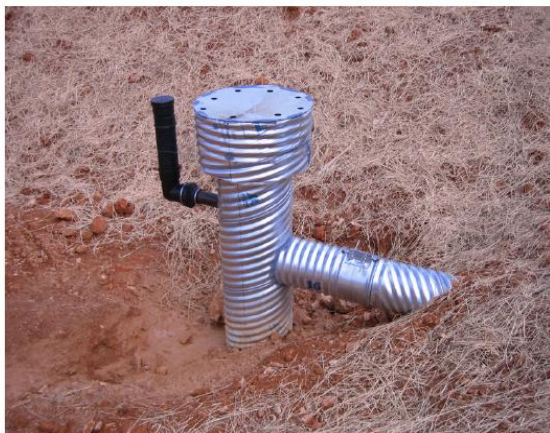
Figure 7.31-6 Dewatering device on Riser with Trash Rack
